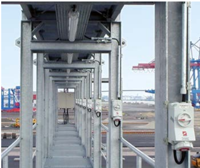
Container Terminal, Altenwerder – Germany
