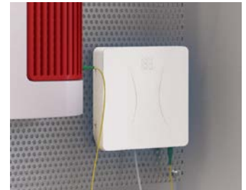
Example: Installation in the multimedia distributor.
