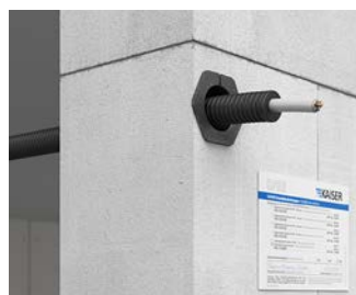
Wall feed-through in sand-lime brick fire-protection wall.
