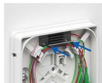
Perform splicing work and place the crimp splice protector in the holder.
