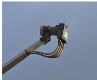
4 coaxial cables are connected here for reception.
