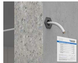
Wall feed-through in concrete fire-protection wall.
